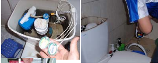
For flush toilet Installation of a counter and measurement of flushing volume
